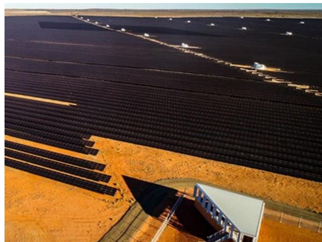
Image: Broken Hill Solar Plant.
